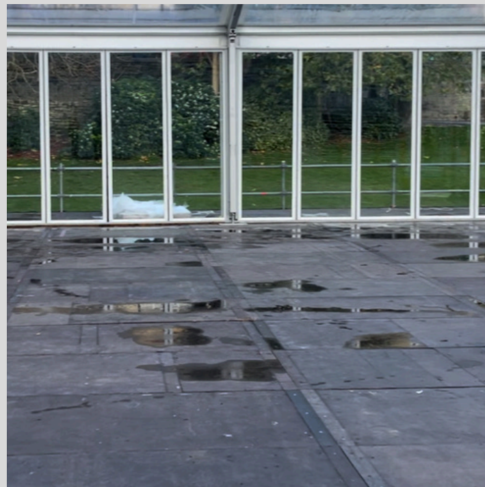
Glass marquee panels
